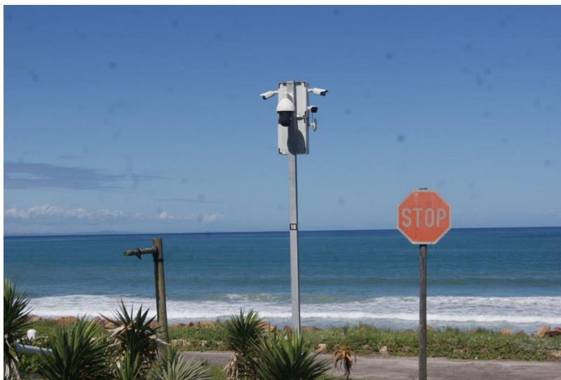
Figure 2 Typical CCTV pole
