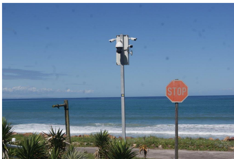
Figure 2 Typical CCTV pole
